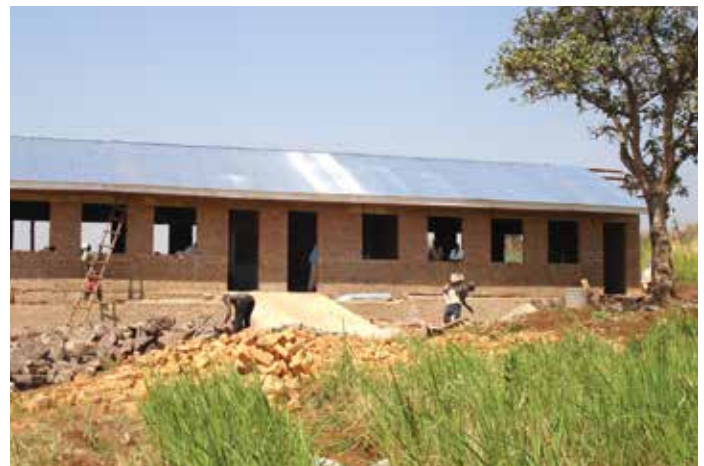
New block for Kababiito Early Childhood Development Centre, built in 2014 thanks to the generosity of CFTC donors like you!
